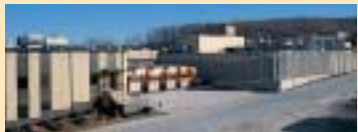
INDUSTRIAL BATTERY PLANT
